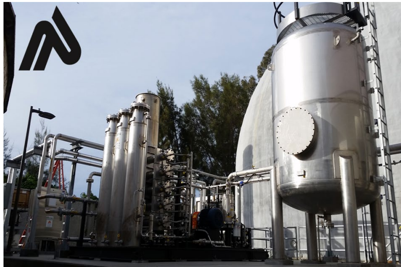
Figure 3-5. DG upgrading system at San Mateo WWTP (California) using Unison’s BioCNG system Includes H 2 S removal, moisture removal, compression, siloxane removal, and membrane separation.
