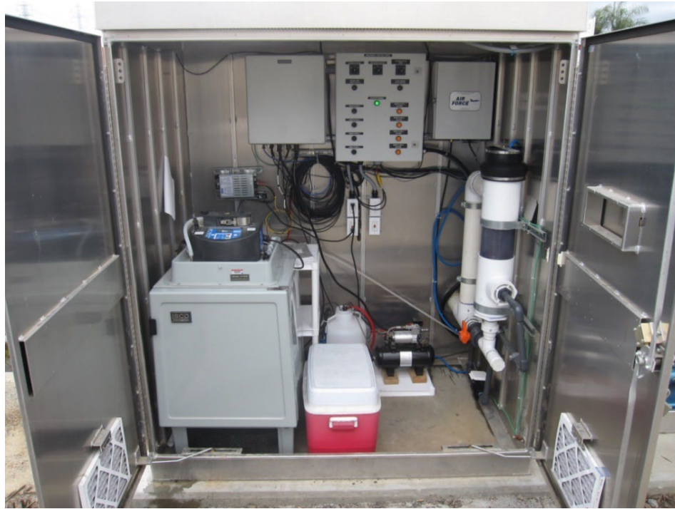
Figure 4-3. Example of pH monitoring station for EHB or septage receiving
