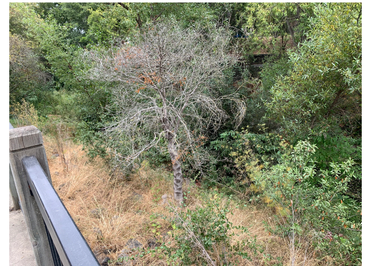
Santa Rosa Creek Heavy vegetation on banks - visibility to stream bed obscured by vegetation
