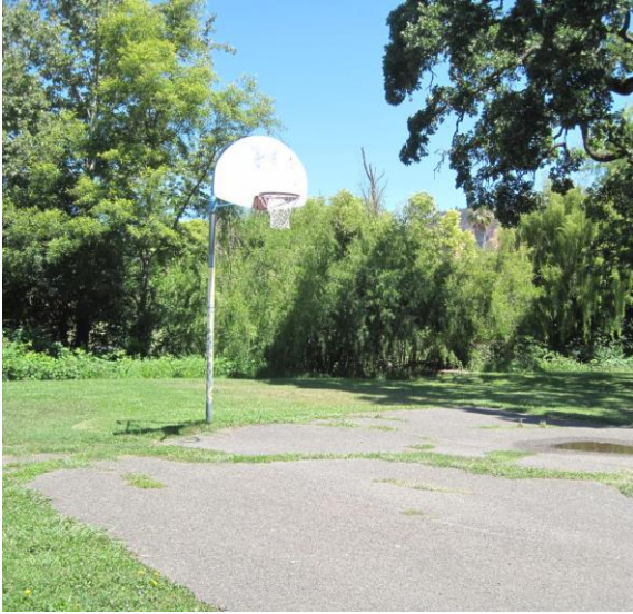
Cracks and weeds in surfacing. Potential trip hazard.
