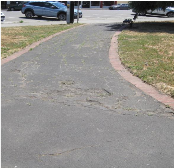
Cracks and potholes creating uneven surfacing.
