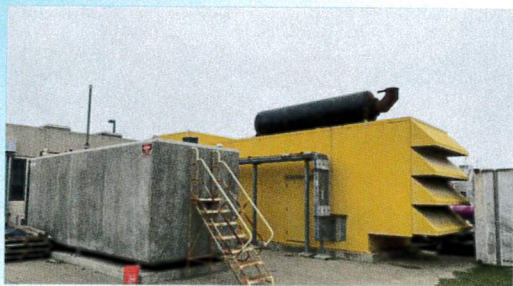
Tracy WWTP emergency generator diesel fuel tank with containment.
