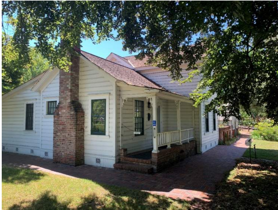
Current image of west elevation of Main House. Another alteration to the drainage system is that the existing wood box gutter integral to the cornice has been shingled over at this location.
