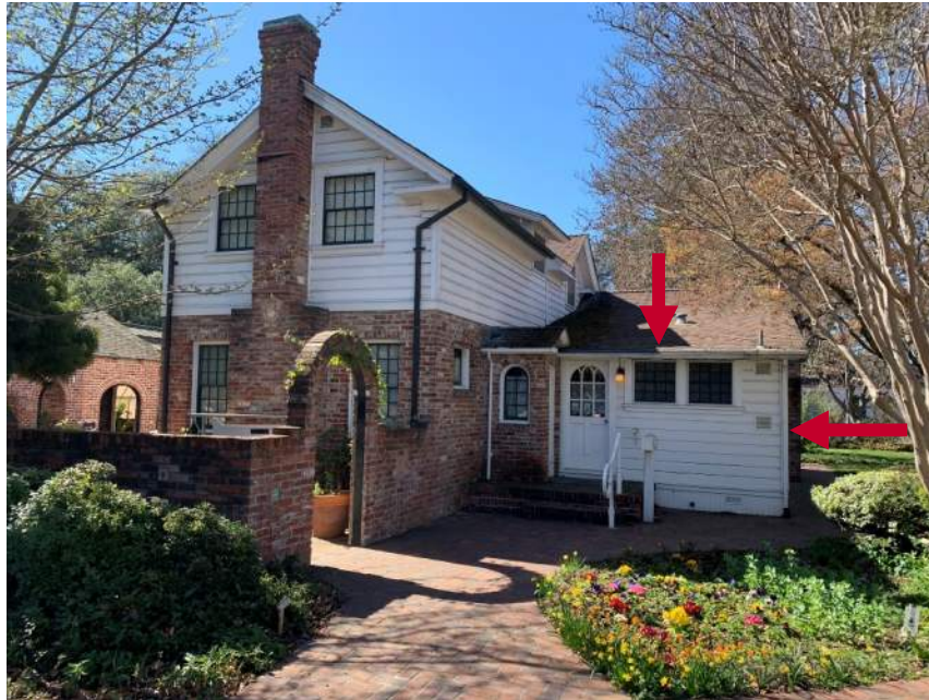
Current image of rear (east) elevation of Main House. Note the existing asphalt roofing is a red-brown color. One alteration to the gutters and downspouts is the installation of a new gutter and downspout on the east elevation (red arrows). This newer gutter and downspout replaced the existing wood box gutter integral to the cornice that was shingled over and abandoned at this location.
