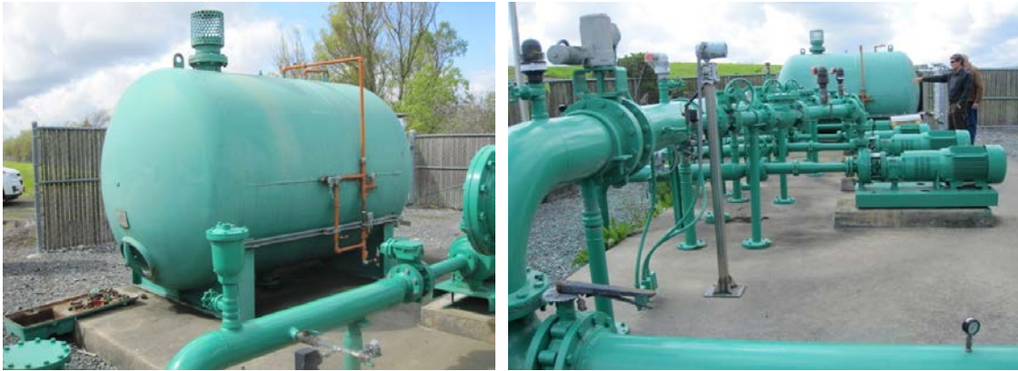
Figure 3-3: Disconnected Hydropneumatic Tank at Todd Road Pump Station
