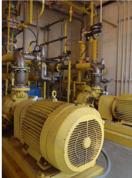
Figure 1-10: Digester Gas Mixing Pumps
