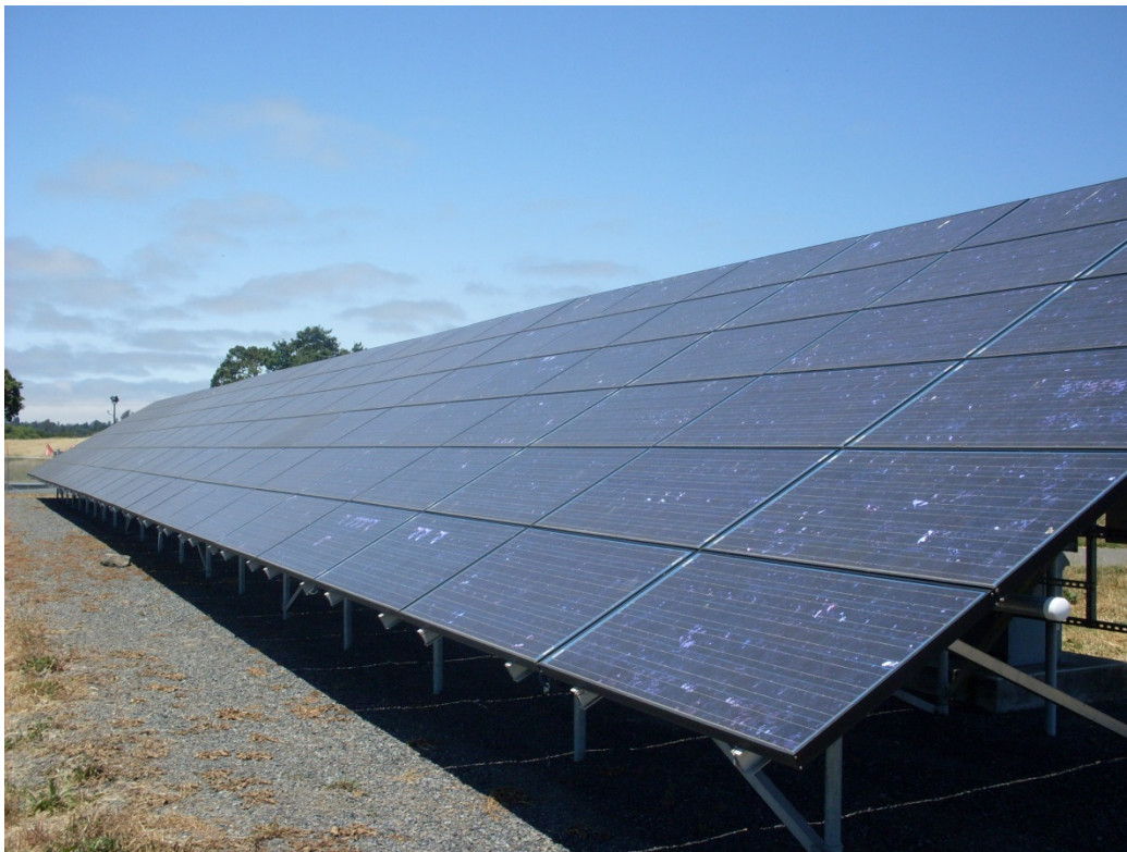
Figure B-1: Fixed Tilt System Installed at Laguna Treatment Plant
