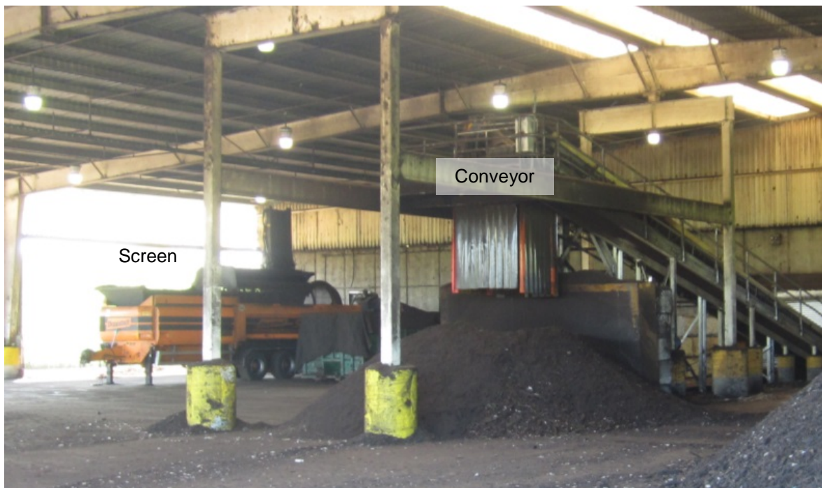
Figure 2-5: Screening Equipment Location Relative to Conveyor
