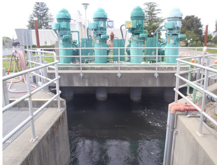
Figure 1-3: Tertiary Filter Wet Well Pumps
