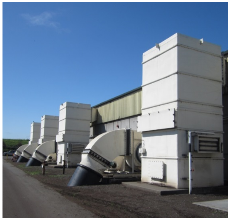
Figure 2-3: Compost Building Exhaust Fans
