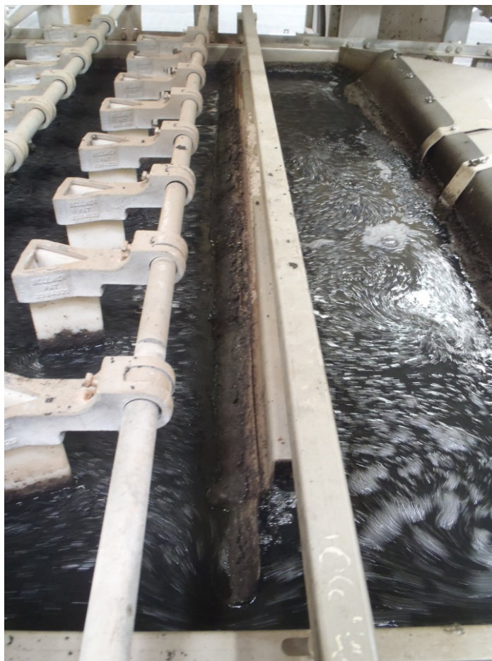
Figure 1-13: Belt Press Equipment
