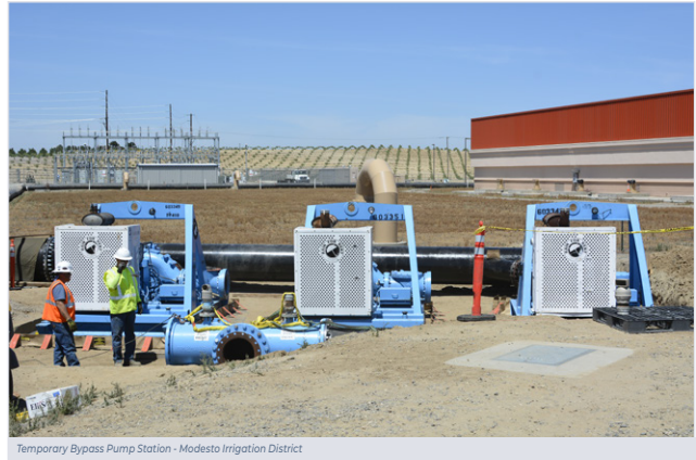
Temporary Bypass Pump Station - Modesto Irrigation District
