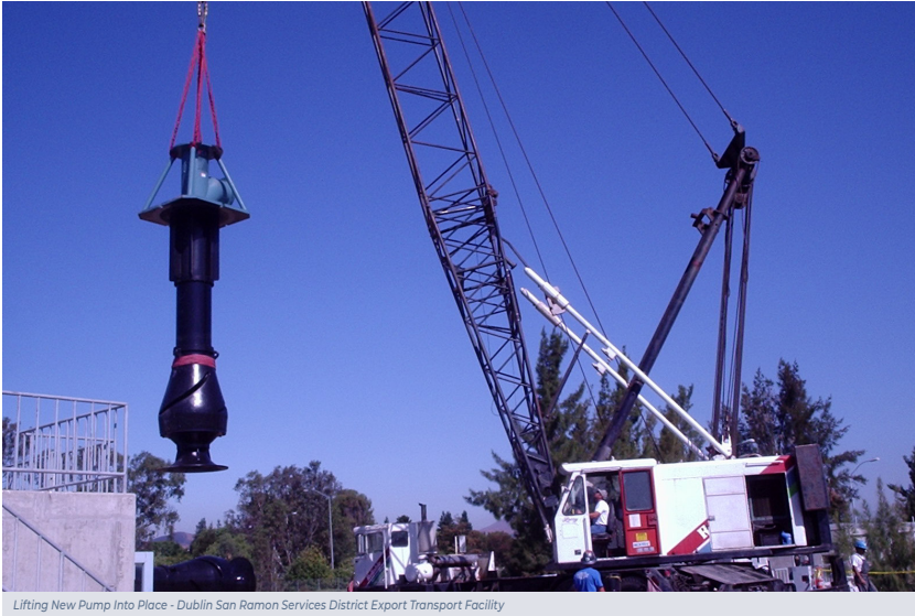
Lifting New Pump Into Place - Dublin San Ramon Services District Export Transport Facility
