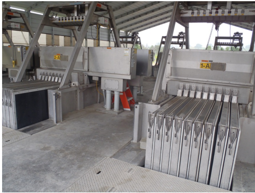
Figure 1-4: UV Disinfection Equipment
