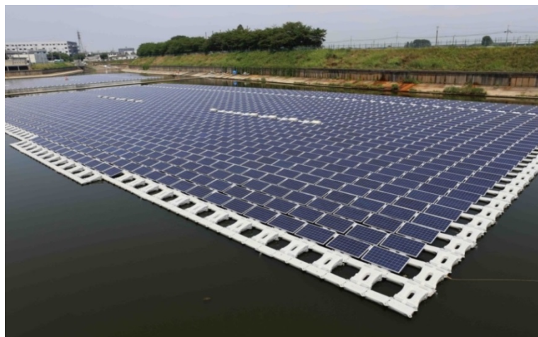
Figure B-3: 1.2 MW Flotovoltic System Installed in Okegawa, Japan
