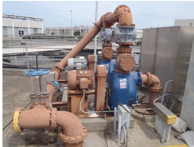
Figure 1-9: RAS Pumps Adjacent to the Clarifier
