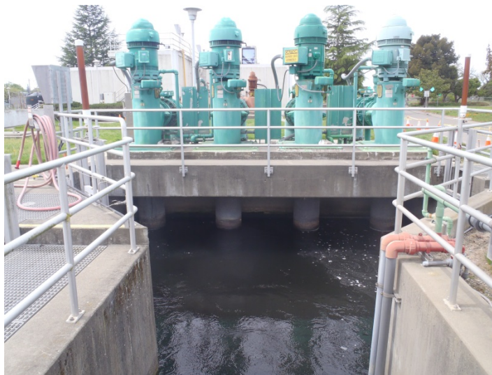
Figure 1-3: Tertiary Filter Wet Well Pumps
