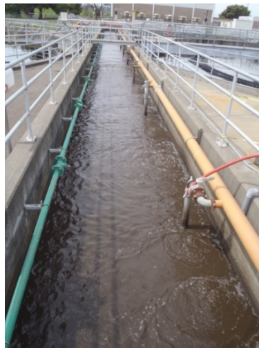
Figure 1-7: Mixed Liquor Channel with Aeration
