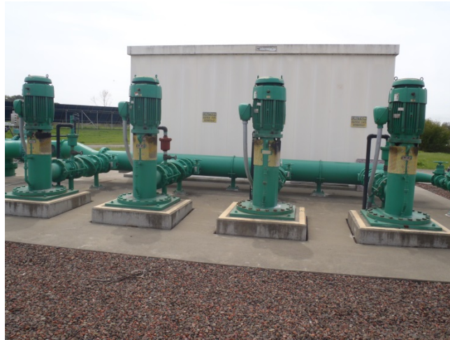
Figure 1-6: Recycled Water (3W) Booster Pumps
