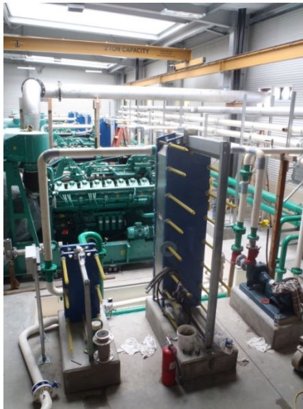
Figure 1-8: Overview of the CHP Facility
