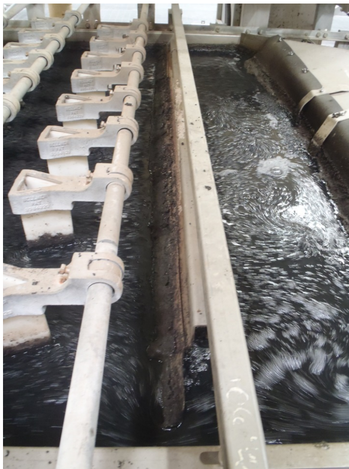
Figure 1-13: Belt Press Equipment
