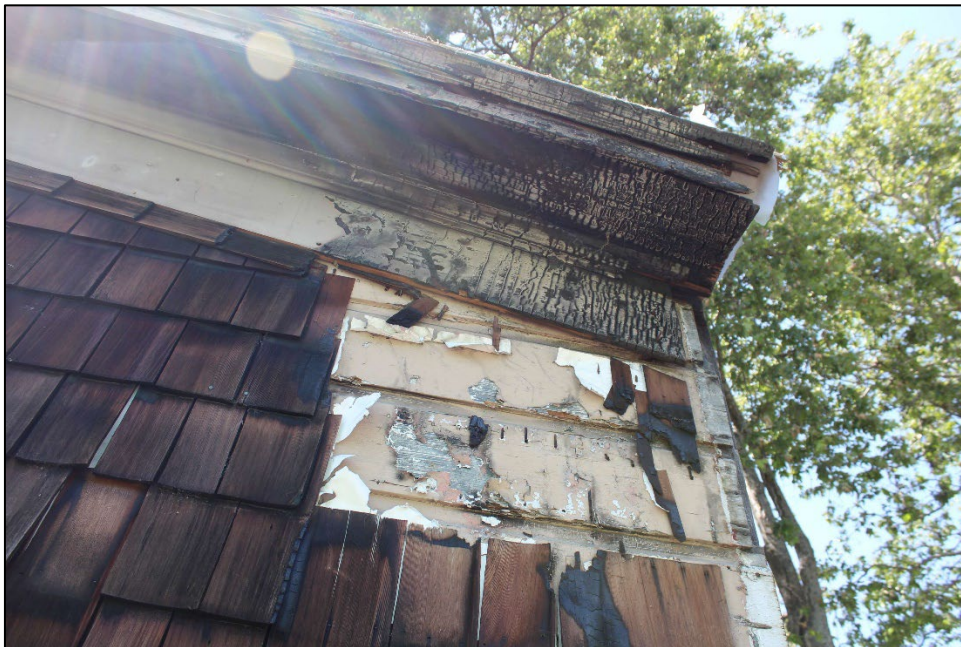
Photo 11: Fire damage, northeast corner
