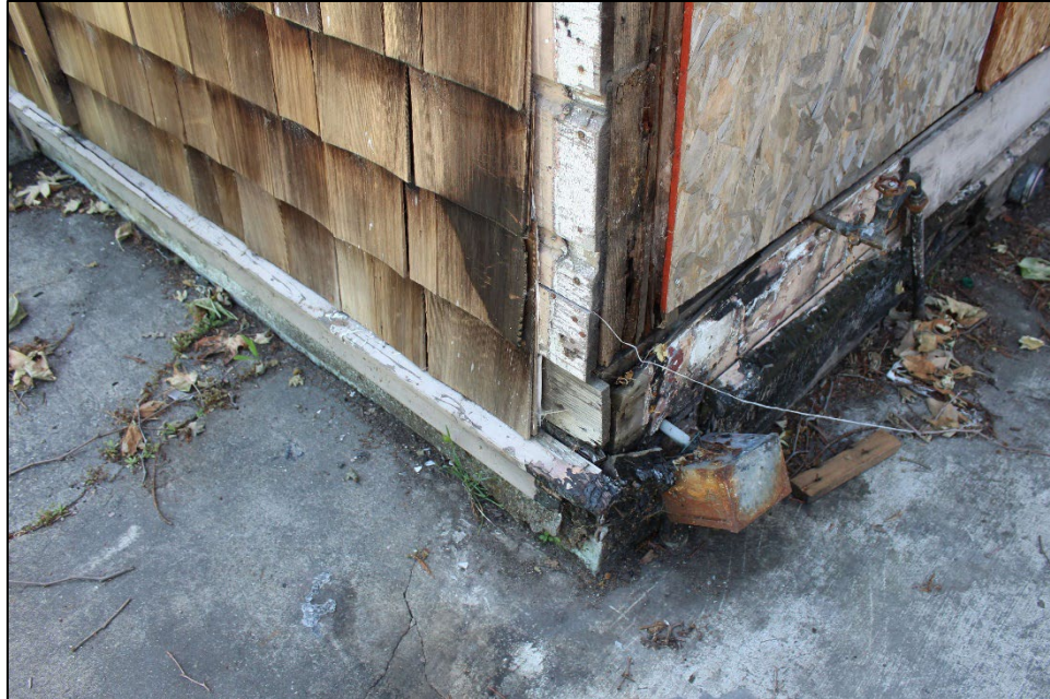
Photo 10: Fire damage, northeast corner
