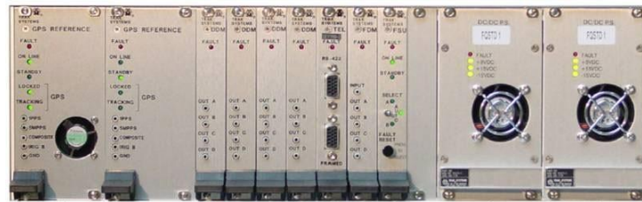
Figure 1-11: TRAK 9100 Simulcast Site Reference –Provides the simulcast system 1 PPS, 5 MPPS, and 1 PPS + 5 MPPS composite signals to synchronize the simulcast transmissions
