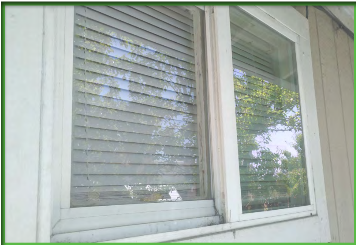
H. Newly Installed Dual Pane Windows in Good Condition with Minimal Maintenance Issues (Permit for Inserts Not Required)
