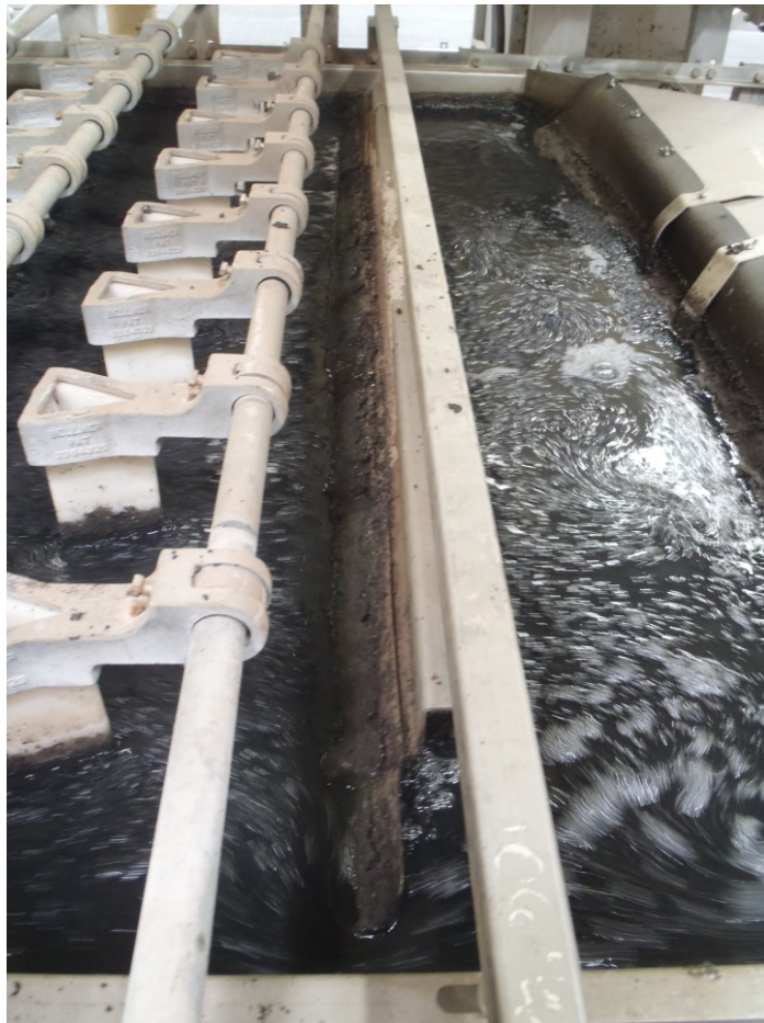
Figure 1-13: Belt Press Equipment
