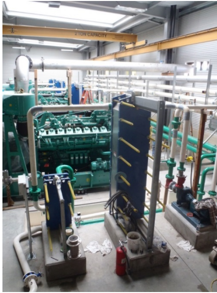
Figure 1-8: Overview of the CHP Facility
