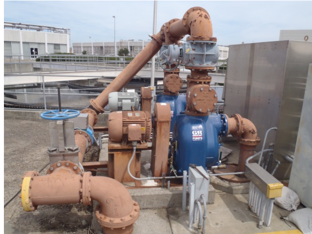
Figure 1-9: RAS Pumps Adjacent to the Clarifier
