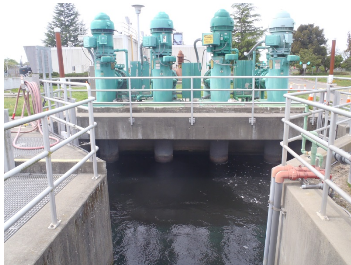
Figure 1-3: Tertiary Filter Wet Well Pumps
