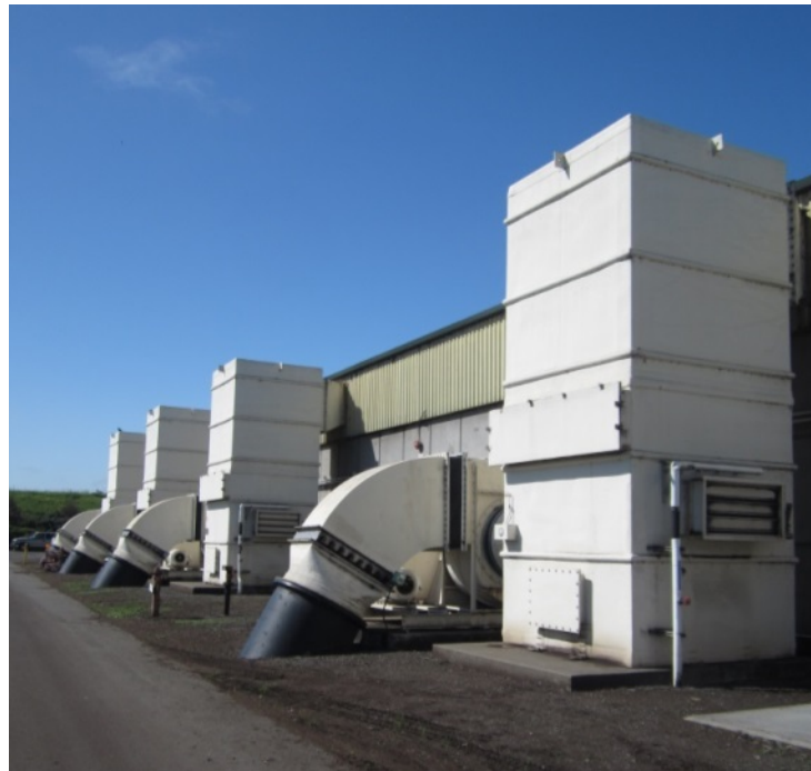
Figure 2-3: Compost Building Exhaust Fans
