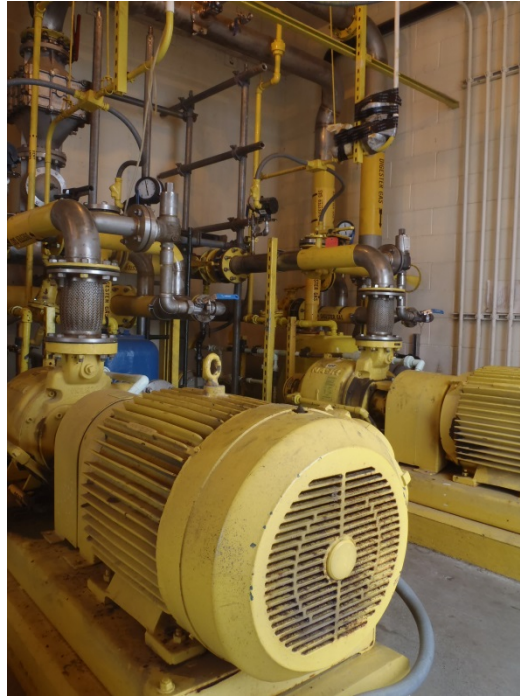
Figure 1-10: Digester Gas Mixing Pumps
