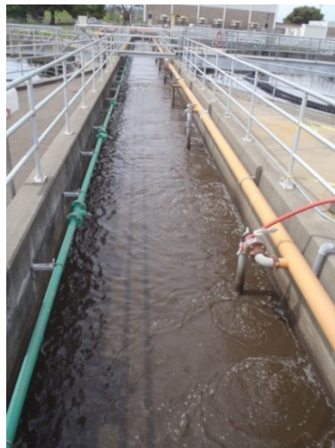
Figure 1-7: Mixed Liquor Channel with Aeration
