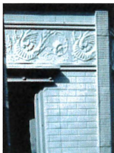
Decorative pressed metal interior or exterior features should not be cleaned abrasively. Photo: NPS files.
