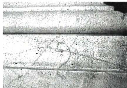
Very high-pressure water has scarred this granite. Photo: NPS files.
