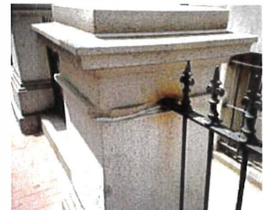
The iron stain on this granite post may be removed by applying a commercial rust-removal product in a poultice. Photo: NPS files
