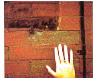
Undamaged historic brick (above). Sandblasted brick (below). Photo: Courtesy, Illinois Historic Preservation Agency.
