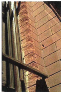
Brick molding next to the window has been severely abraded by sandblasting to remove paint. Photo: NPS files.
