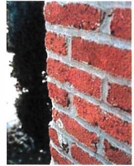
Abrasive cleaning can cause permanent damage to historic fabric, such as this brick wall. Photo: NPS files.
