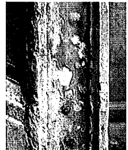
This clear coating has failed and is pulling off pieces of the stone as it peels. Photo: NPS files
