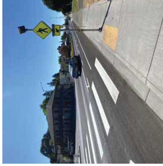
Figure 25. Rectangular Rapid-Flashing Beacon in Santa Rosa
