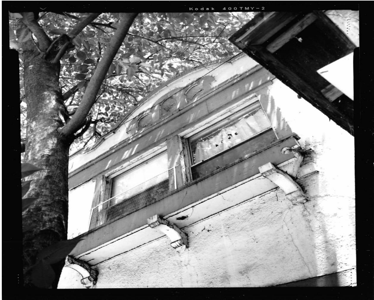
608 Morgan Street - Photo #3 - EXTERIOR; DETAIL OF SECOND FLOOR WINDOW PAIR WITH BLIND ARCHES, WOOD WINDOW SURROUND, AND WOODEN FLOWER BOX WITH BRACKETS, VIEW TO NORTH.
