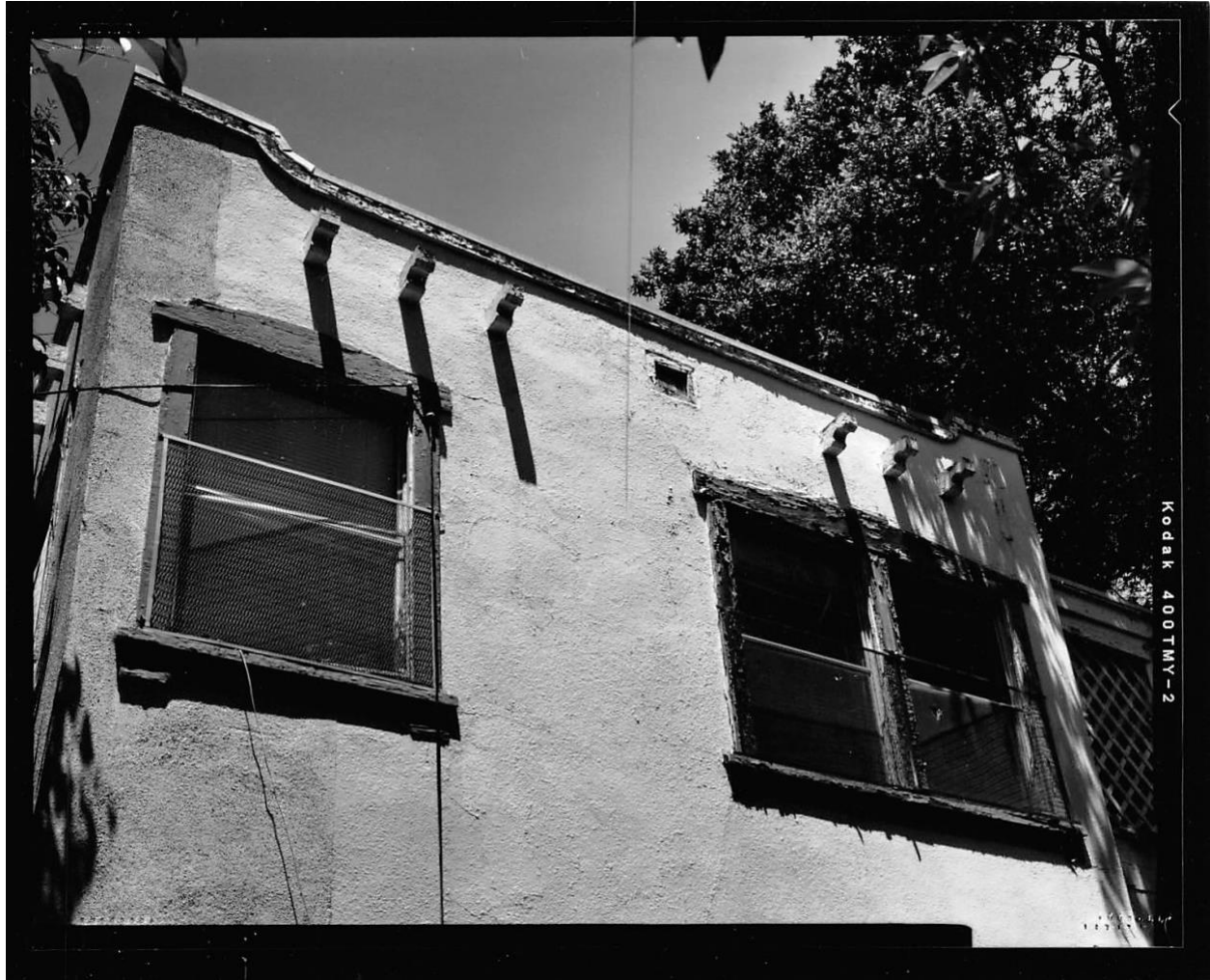
608 Morgan Street - Photo #7 - EXTERIOR; DETAIL OF SECOND FLOOR WINDOWS, INCLUDING WOOD WINDOW SURROUNDS AND PROJECTING VIGAS; VIEW TO THE NORTH.
