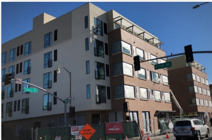
AC Hotel by Marriott construction as seen from the intersection of Davis and Fifth Street
