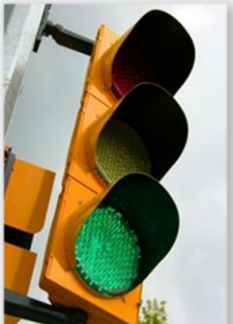
214 Traffic Signals 81 Pedestrian Flashers
