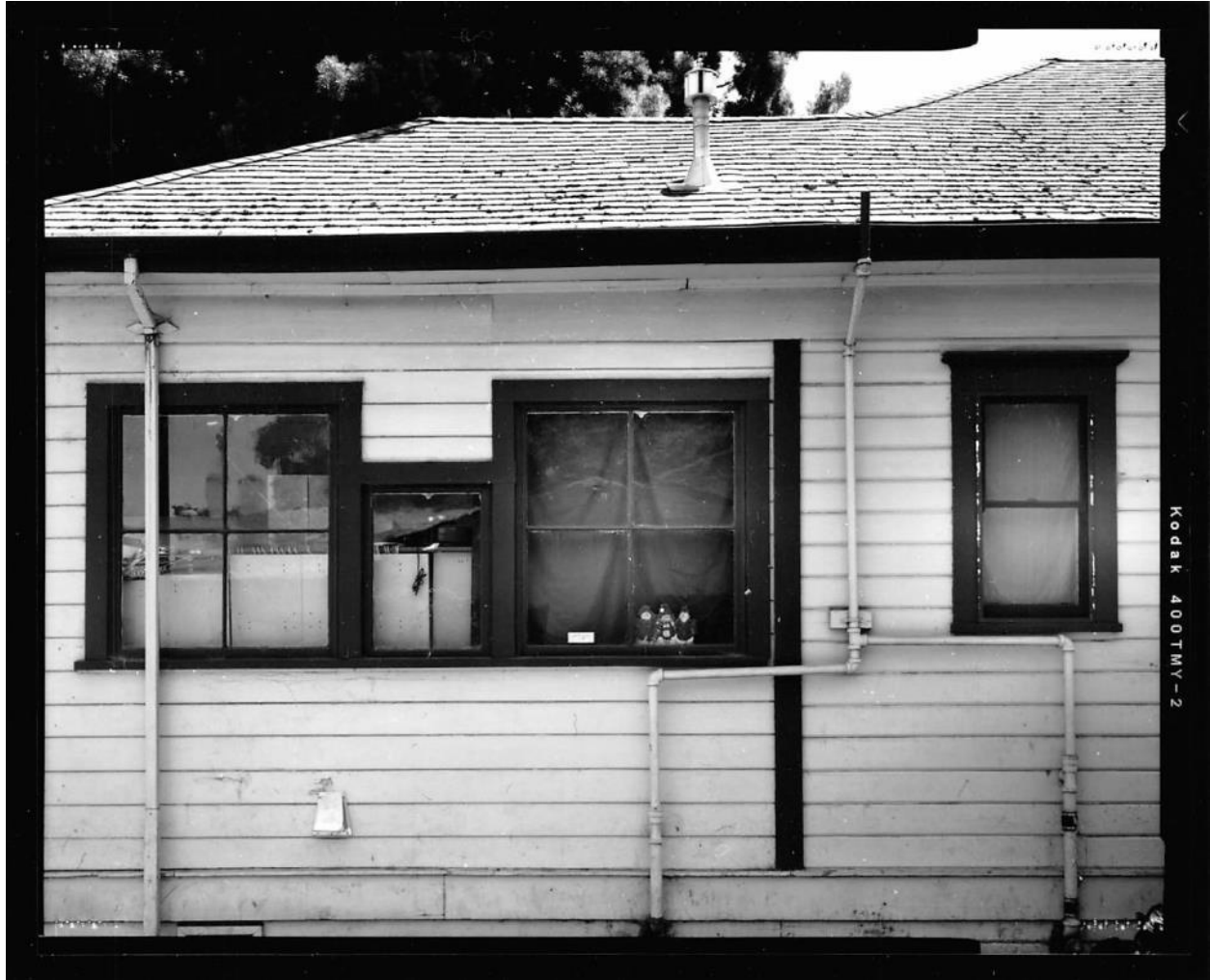
520 Morgan Street - Photo #7 - EXTERIOR, DETAIL OF NORTH (SECONDARY) FAÇADE WINDOW GROUPING, VIEW TO SOUTH.
