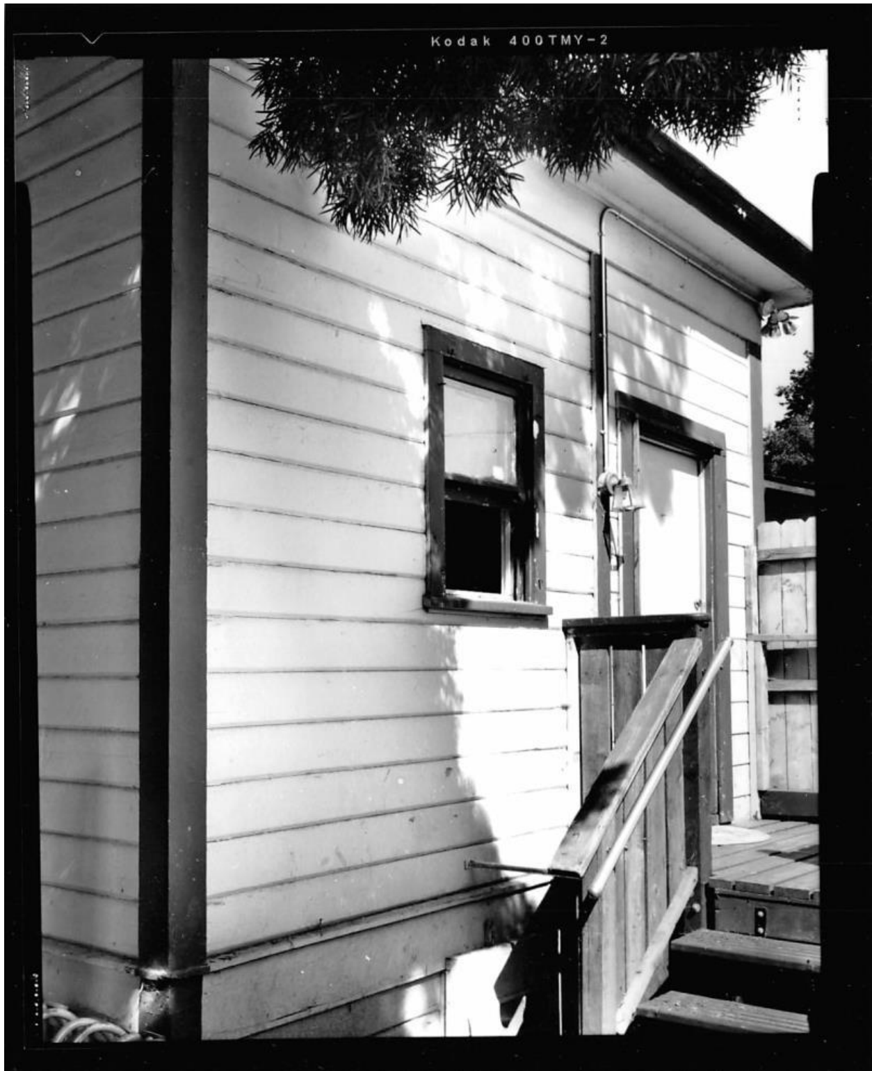
520 Morgan Street - Photo #5 - EXTERIOR, DETAIL OF EAST (REAR) FAÇADE ENTRY, VIEW TO WEST.
