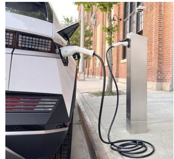
It's Electric EV Charging Station
