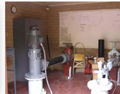
20 Pump Stations 17 Sewer Lift Stations
