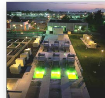
Laguna Treatment Plant
