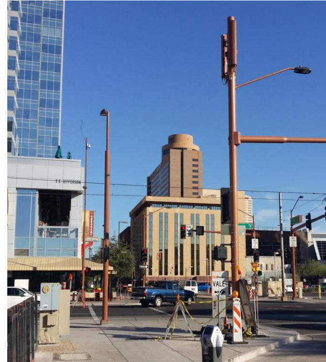
Traffic Control Pole with Cabinet
