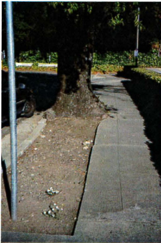
Tree root damage and a barren garden strip at 6 th and Davis.
