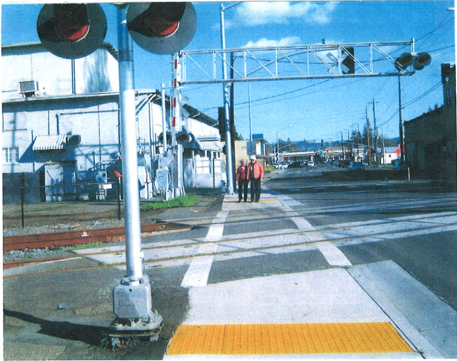
Guerneville Rd. sidewalk double-track Crossing with no pedestrian gates (1/31/16)
