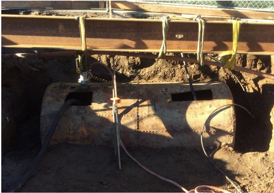
Abandoned heating oil tank
