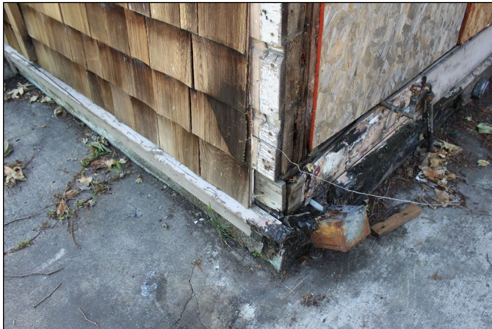
Photo 10: Fire damage, northeast corner
