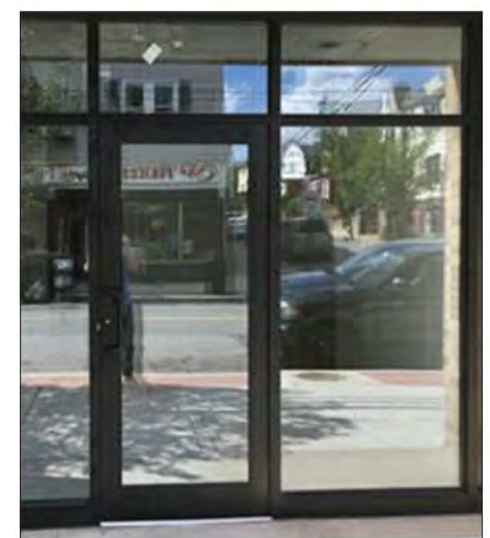
7 ALUMINUM WINDOW STOREFRONT SYSTEM - DARK BRONZE WITH CLEAR AND OPAQUE GLAZING & METAL FASCIA TO MATCH
