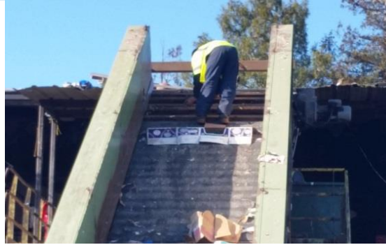
5) Broken Infeed Conveyor at 34000 Standish MRF
