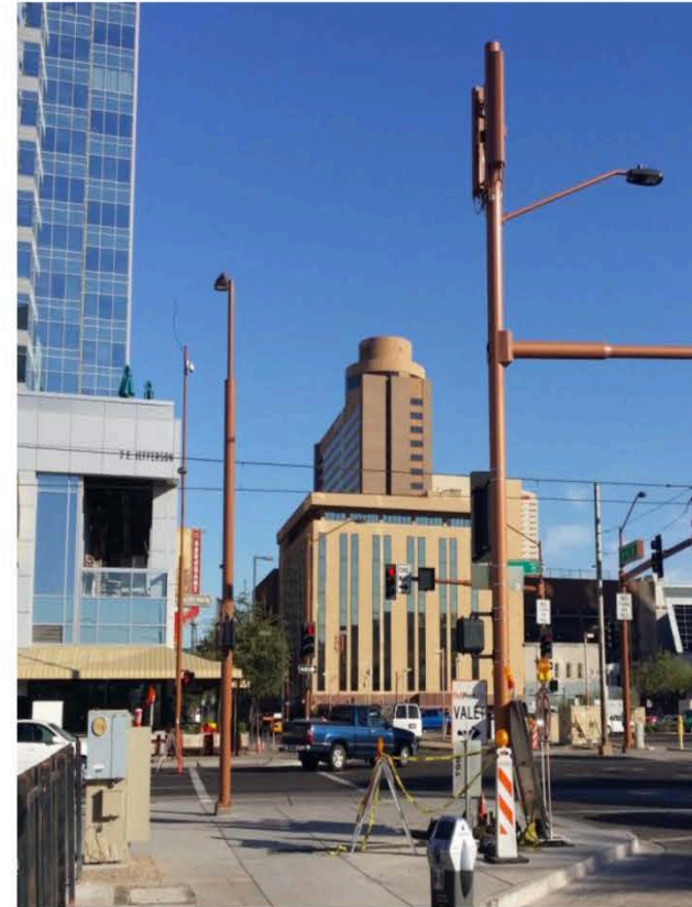
Traffic Control Pole with Cabinet
