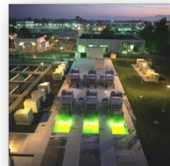
Laguna Treatment Plant
