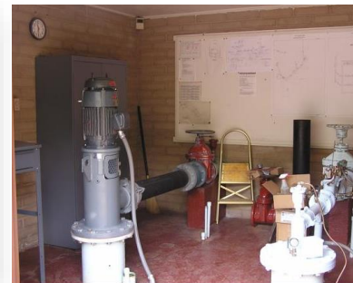
20 Pump Stations 17 Sewer Lift Stations
