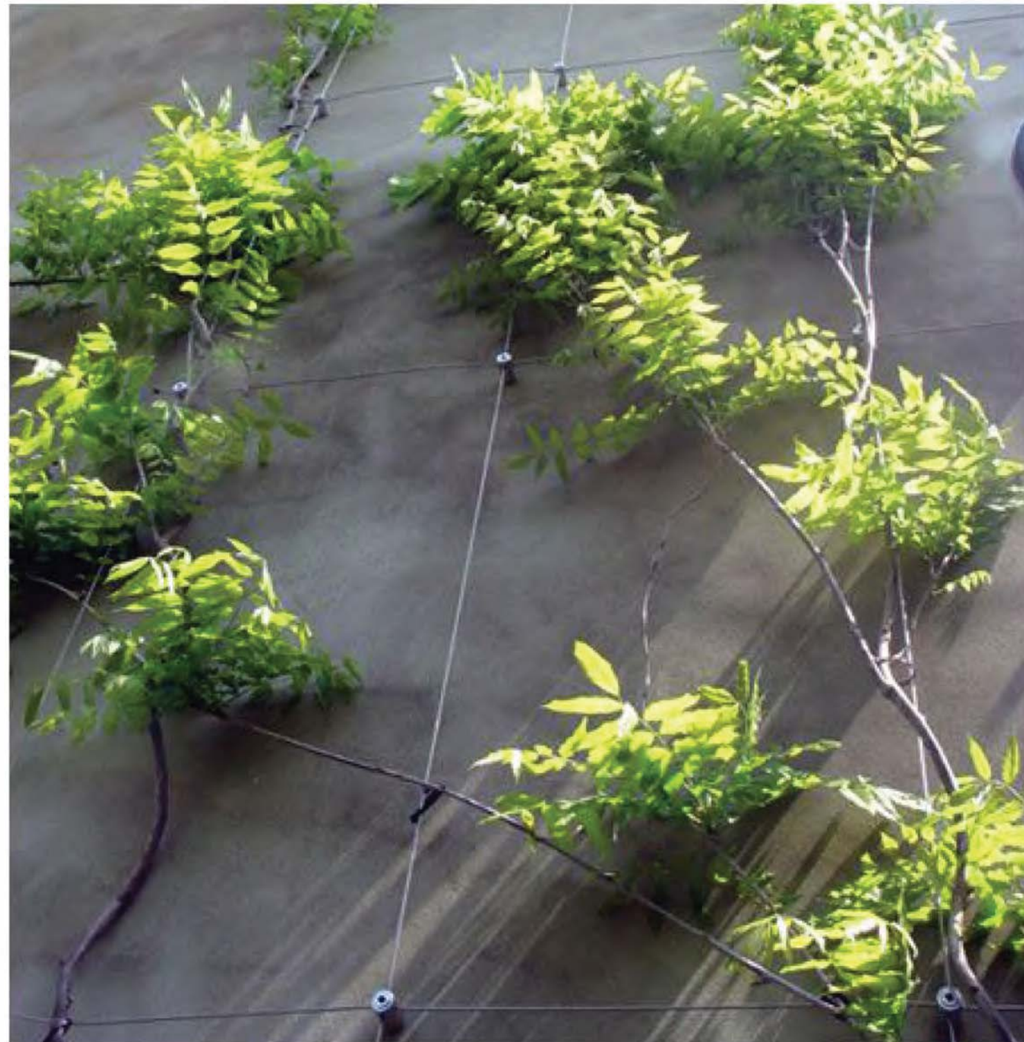
STEEL WIRE TRELLIS FOR VINES
