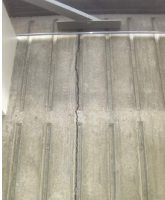
Figure 30: Large Crack Found in Building 5/6/7
