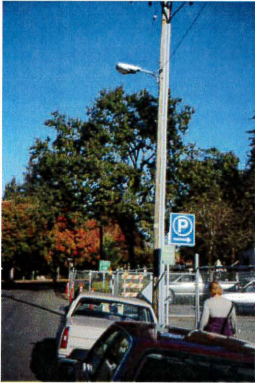
Streetlights as an appendage to a power pole typical of the Cherry Street, St. Rose, and West End neighborhoods.
