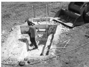
Workers removed the tile and plaster surfaces from the West Recreation Center spa, left, and pool last month prior to refinishing the two.
