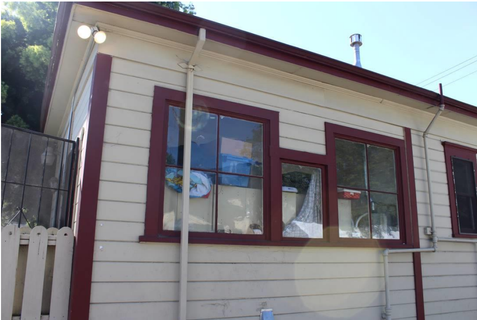
Photograph 6: Detail, windows on northwest elevation, camera facing southeast, April 1, 2016.
