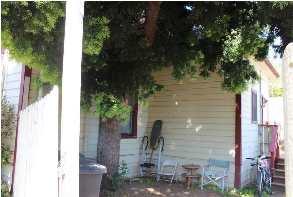
Photograph 4: Northeast elevation, including southeast and northeast elevations of projection, camera facing west, April 1, 2016.
