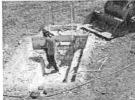
Workers removed the tile and plaster surfaces from the West Recreation Center spa, left, and pool last month prior to refitting the two.
