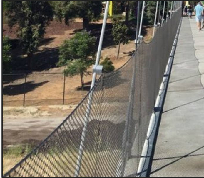
Cable mesh infill attached to cable stays on Happy Hollow Bridge in San Jose, CA
