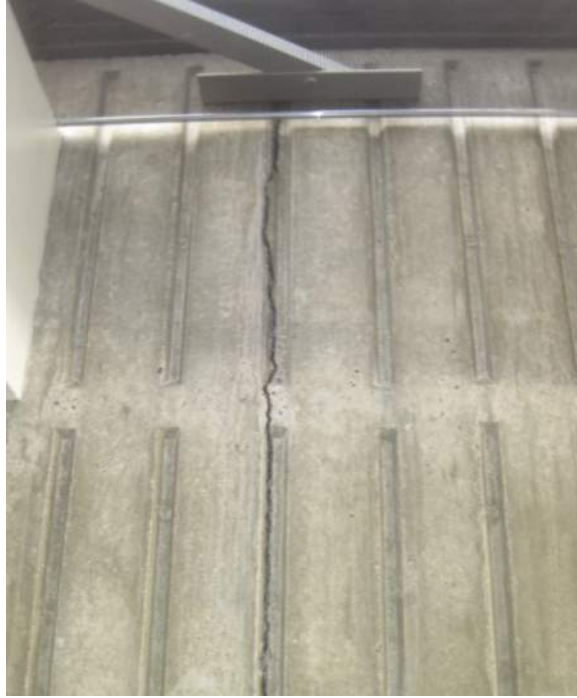
Figure 30: Large Crack Found in Building 5/6/7
