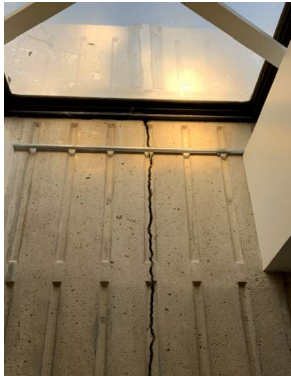
Figure 29: Large Crack Found in Building 3/4
