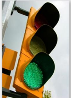
214 Traffic Signals 81 Pedestrian Flashers
