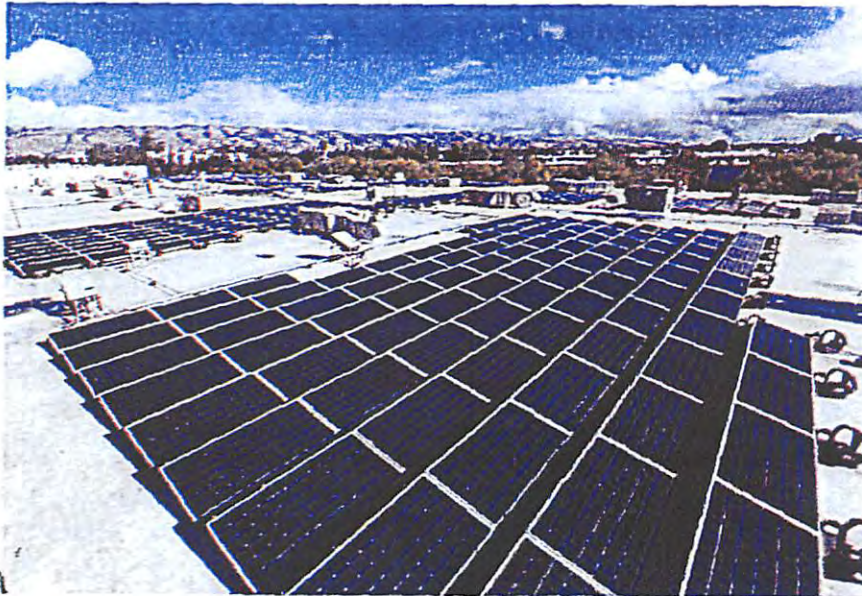
Sprig Electric HQ PV/Battery Storage Project – San Jose, CA
