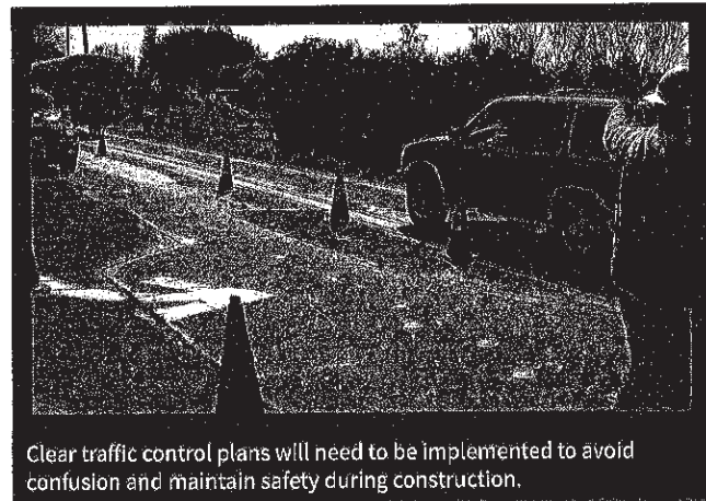
Harris will look out for any sidewalk closures on Stony Point Road to verify pedestrians have an alternate means of access throughout the site. This was a topic of discussion at the Harris Construction Management training in January 2015.
