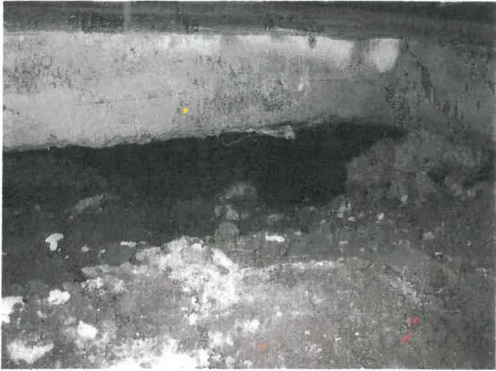
Void under 10-inch slab adjacent to interior footing on east side of building.
