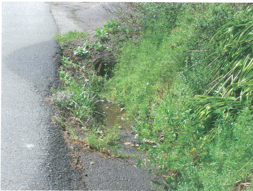
Figure 7. Storm drains would be extended by 27' within the existing ditch on the north side of Chanate Road.
