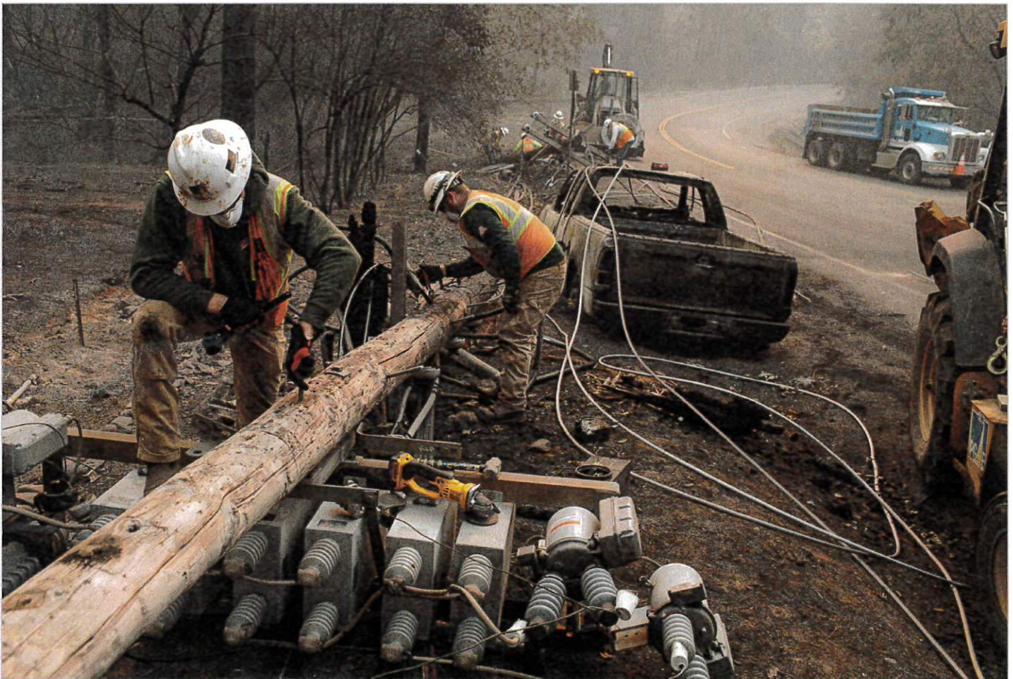
PG&E crews work to replace telephone poles that were burned by the Camp Fire on Billie Road in the town of Paradise in Butte County on Saturday, Nov. 17, 2018, more than a week after the fire broke out. (Kevin N. Hume/S.F. Examiner) PG&E workers disassemble broken power lines after the Camp fire ripped through Paradise, Calif., on Nov. 15, 2018. (Joel Angel Juarez/Zuma Press/TNS)
