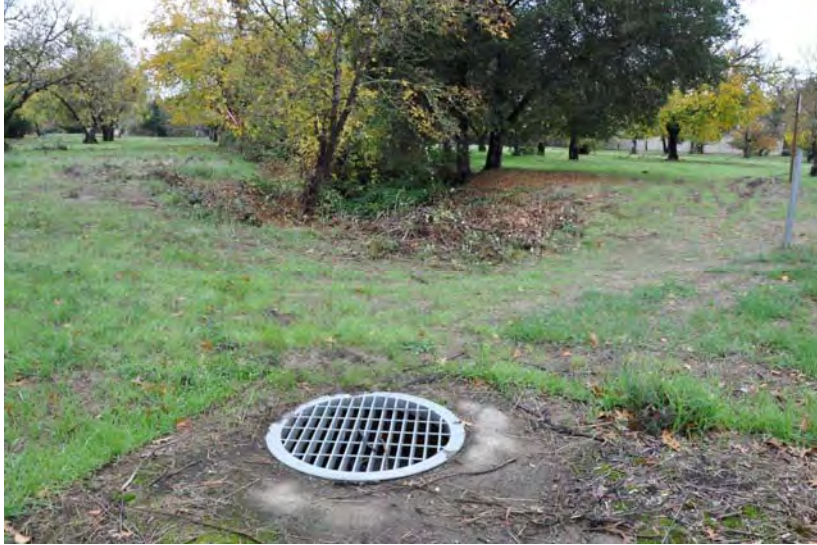
Figure 5: The Spring Creek diversion structure is below this grate. The trees in the middle of the photo are in the old creek channel.
