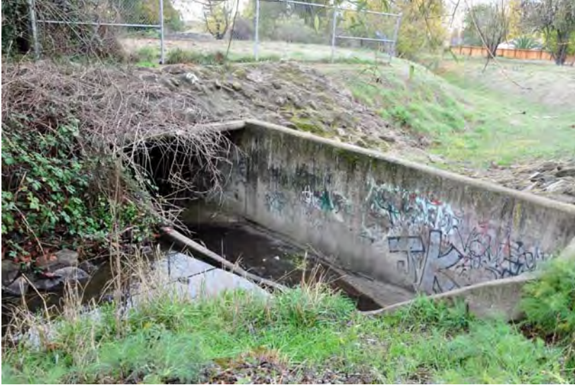
Figure 7: Sierra Park Creek diversion into the Spring Creek Diversion.
