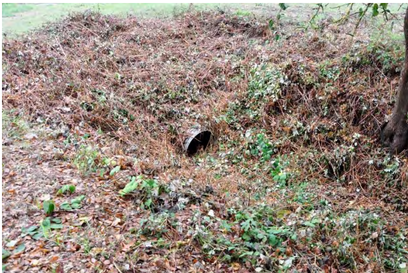
Figure 6: The outfall from the Spring Creek Diversion into the old creek channel note that the bottom of the culvert pipe is filled with sediment.
