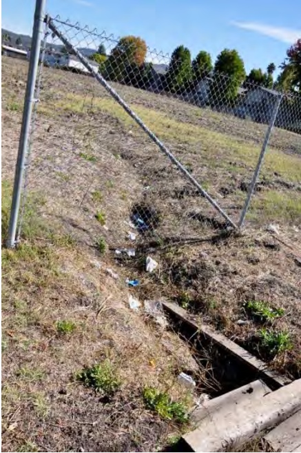
Figure 3: Local site drainage ditch that has collected trash.
