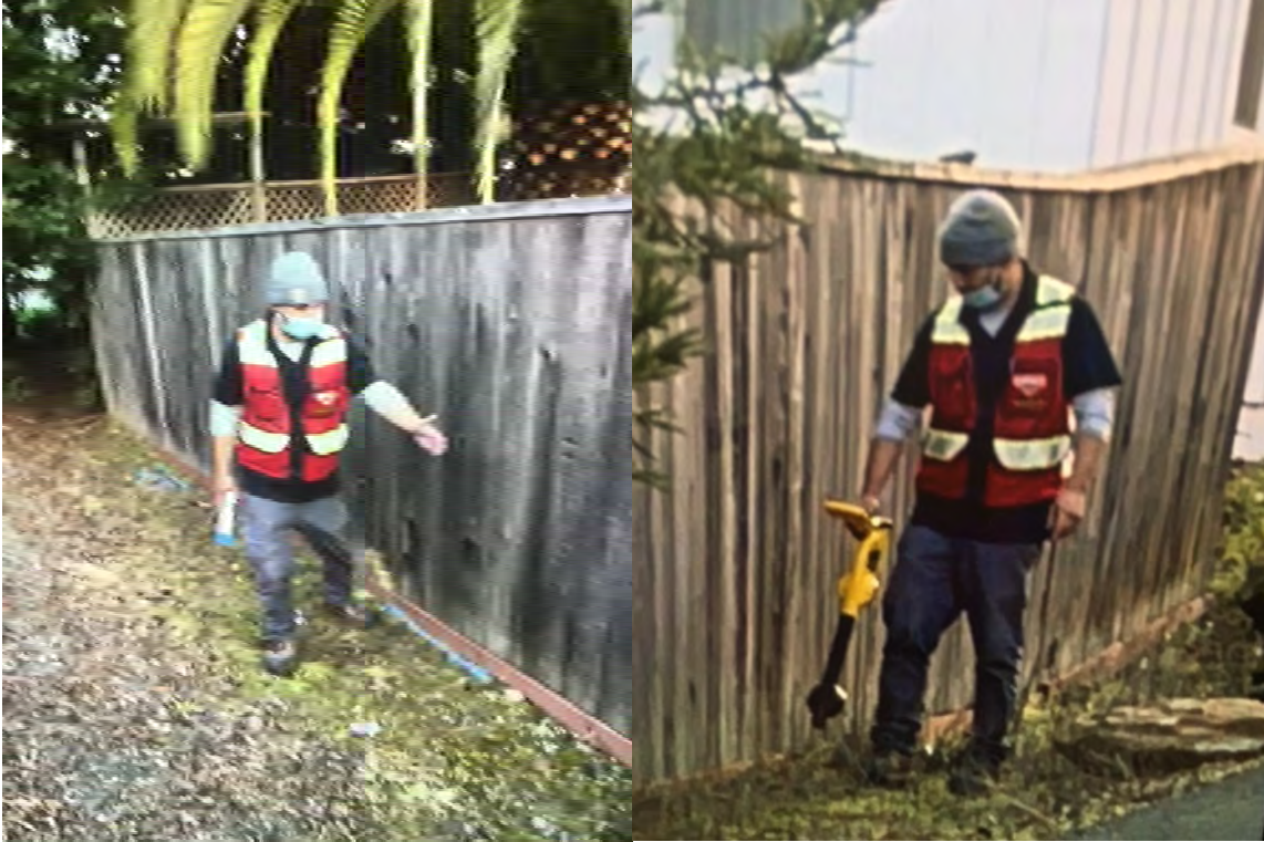
GPRS hired to trace private water line(s) from road. Water line traces along 1900 Brush Creek Fence
