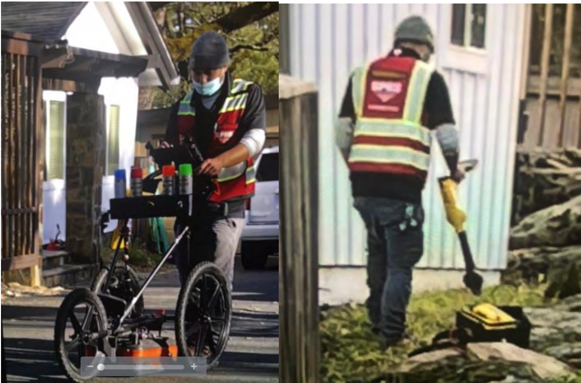
Water line(s) to other homes on private road appear to travel from Brush Creek Rd through 1900 Brush Creek driveway and along-side the new build in the easement and down the 1900 Brush Creek fence line
