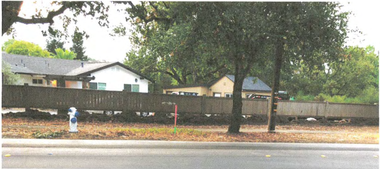
After Unpermitted Excavation of Dirt along Scenic Brush Creek Road
