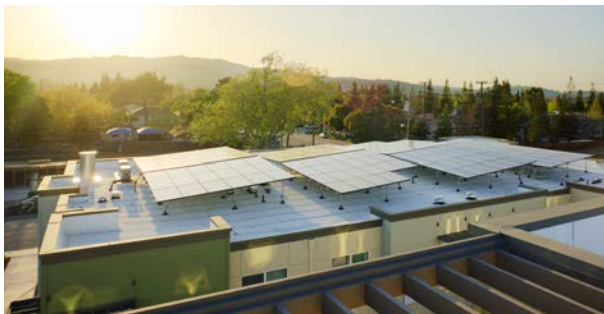
RENEWABLE ENERGY GENERATION
