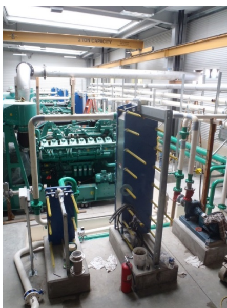
Figure 1-8: Overview of the CHP Facility
