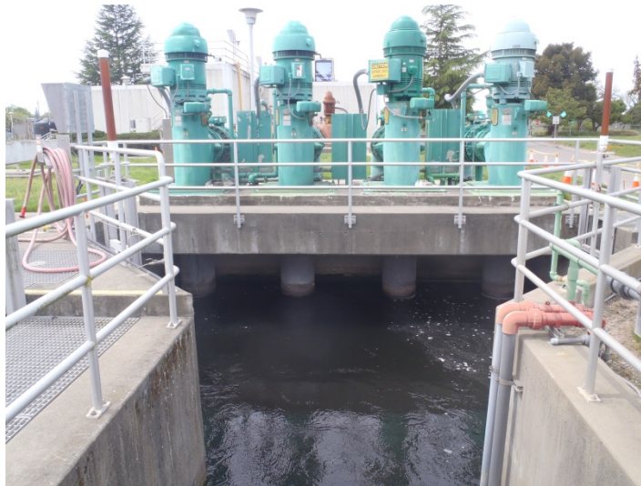
Figure 1-3: Tertiary Filter Wet Well Pumps
