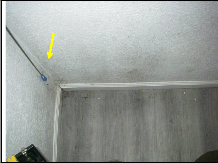
Figure 20. As noted in figure 19, a Swab Sample was taken from the wall in bedroom #3-yellow arrow.
