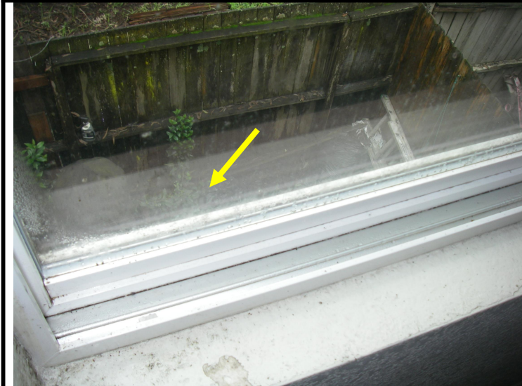
Figure 21. The window sill in bedroom #3 has discoloration and the window pane has condensation buildup-yellow arrow.
