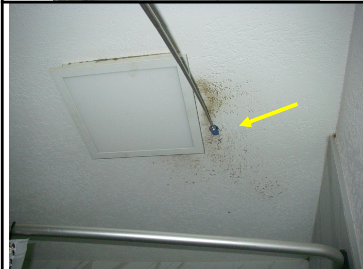
Figure 27. The ceiling in the bathroom has discoloration/possible mold growth and dust buildup. (A Swab Sample was taken from this area).
