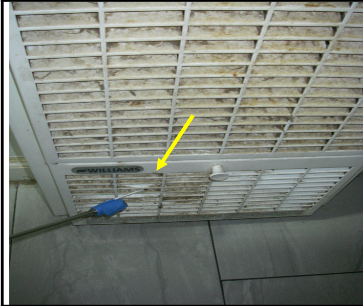
Figure 7. The vent fins of the wall heater of the apartment have dust and possible mold growth. (A Swab Sample was taken from this area - yellow arrow).
