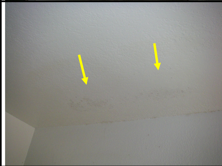
Figure 12. The ceiling by the closet door in bedroom #1 has possible mold growth-yellow arrows.
