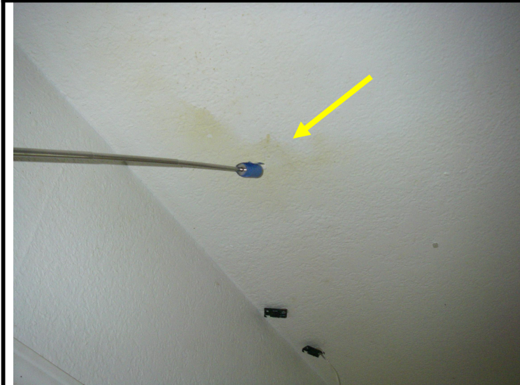
Figure 5. The ceiling above the entry door has discoloration. This condition was also observed in the hallway and kitchen area. (A Swab Sample was taken from this area - yellow arrow).
