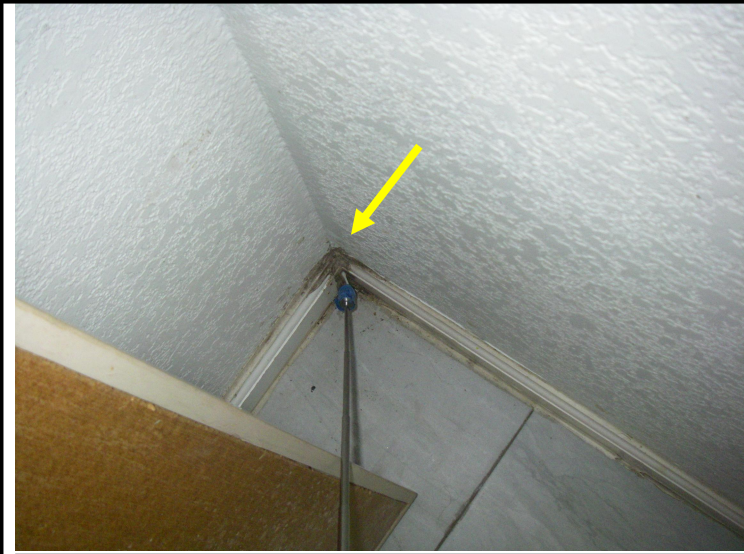
Figure 2. The lower corner wall-to-baseboard transition to the left of the living room sliding glass door has discoloration and probable mold growth. (A Swab Sample was taken from this area-yellow arrow).
