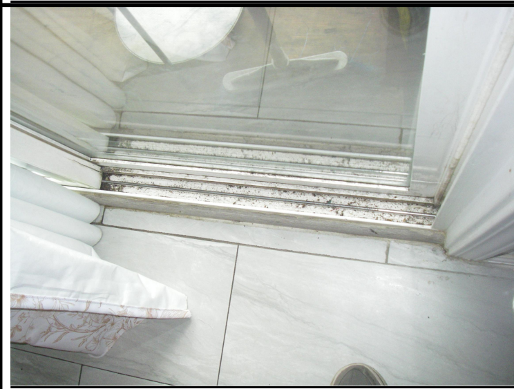
Figure 3. The sliding glass door track in the living room has dust/debris and possible mold growth.
