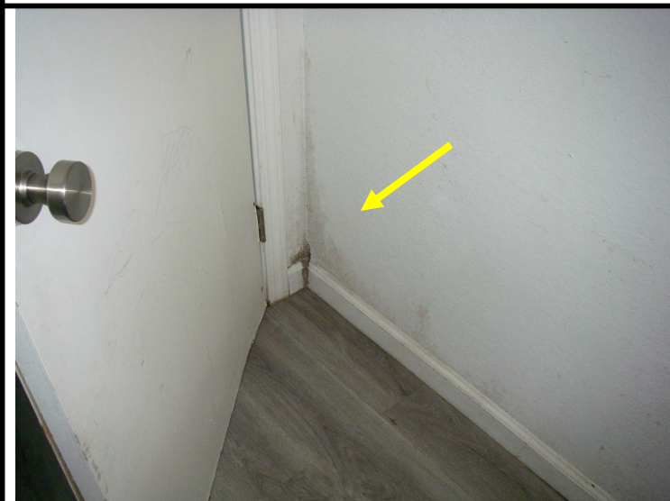
Figure 11. The wall and baseboard behind the door in bedroom #1 has probable mold growth.
