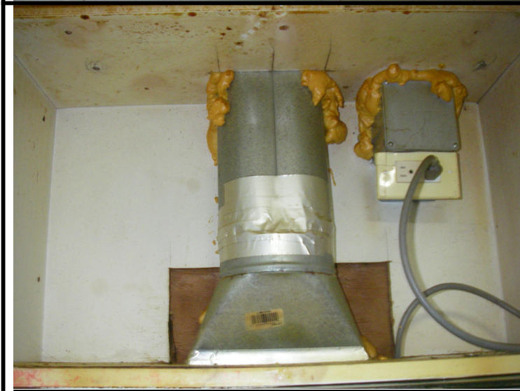
Figure 6. The inside of the cabinet above the microwave has discoloration. This appears to be an accumulation of cooking grease. As previously noted, discoloration was also present on the kitchen ceiling, hallway ceiling and the living room ceiling above the entry door.
