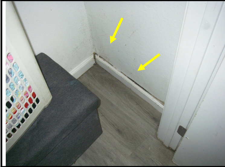
Figure 13. The lower wall and baseboard in the closet in bedroom #1 has probable mold growth.
