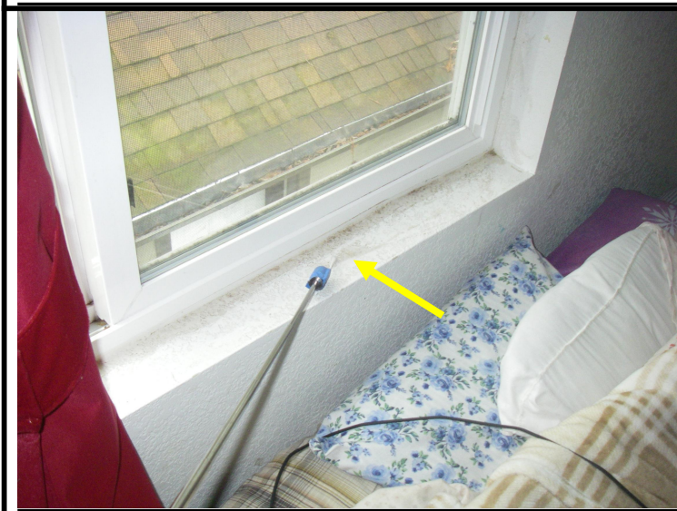
Figure 15. The window sill in bedroom #2 has discoloration/possible mold growth. (A Swab Sample was taken from this area-yellow arrow).
