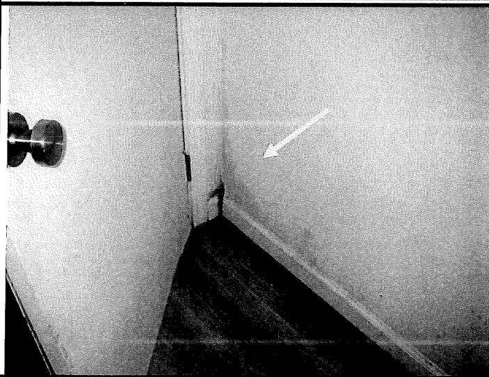
Figure 11. The wall and baseboard behind the door in bedroom #1 has probable mold growth.
