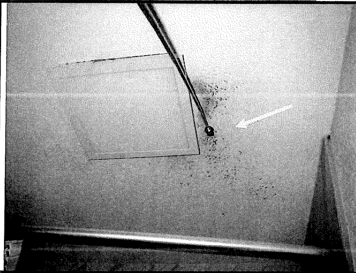
Figure 27. The ceiling in the bathroom has discoloration/possible mold growth and dust buildup. (A Swab Sample was taken from this area).
