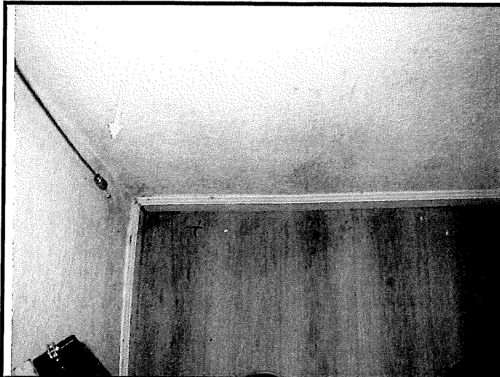
Figure 20. As noted in figure 19, a Swab Sample was taken from the wall in bedroom #3-yellow arrow.
