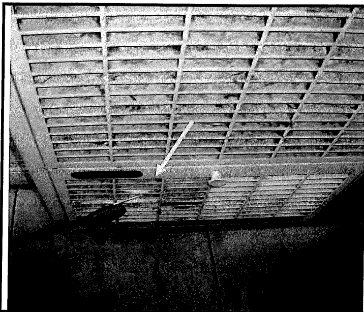
Figure 7. The vent fins of the wall heater of the apartment have dust and possible mold growth. (A Swab Sample was taken from this area - yellow arrow).
