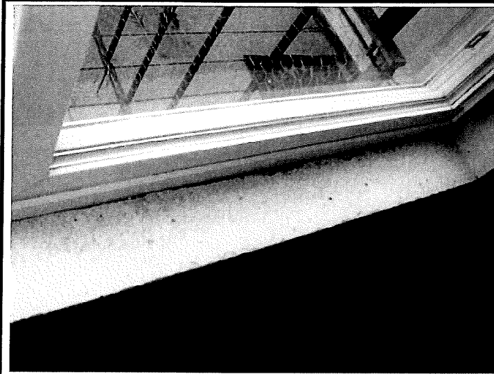
Figure 10. The window sill in bedroom #1 has discoloration/possible mold growth.
