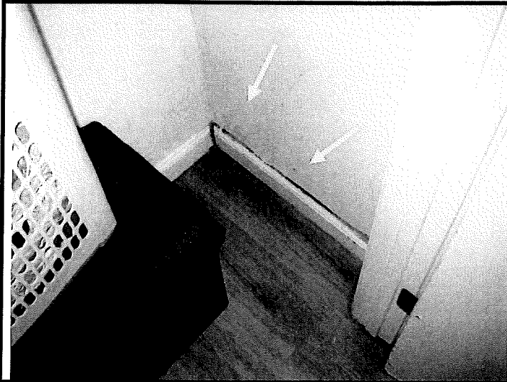
Figure 13. The lower wall and baseboard in the closet in bedroom #1 has probable mold growth.
