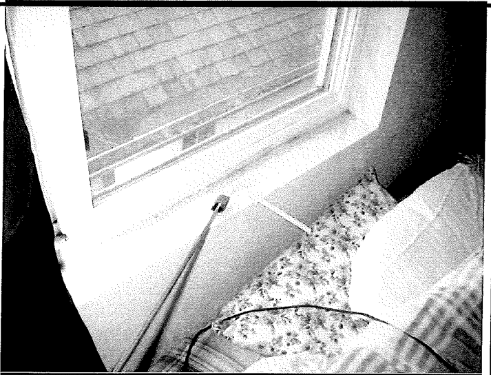
Figure 15. The window sill in bedroom #2 has discoloration/possible mold growth. (A Swab Sample was taken from this area-yellow arrow).
